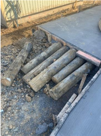
FIGURE 10 TOPPED RETAINING POLES.
